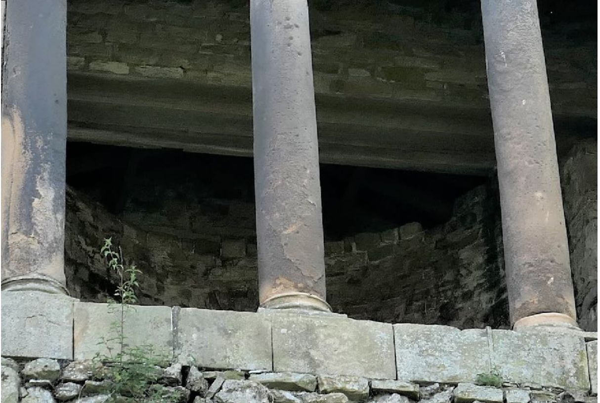
Figure 27. The apsidal wall towards the rear of the 'summerhouse' or folly is only dimly visible from the ground.
