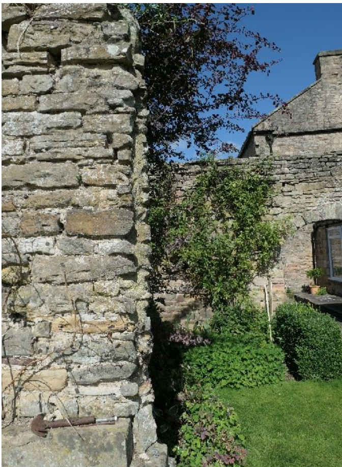
Figure 39. The rebate in the blocking of the mullioned window designed to house the frame of a sash window. The hammer sits on the string course of the plinth believed to have been inserted by Garrett.
