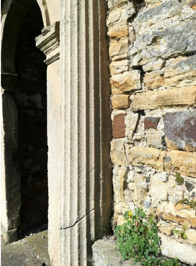
Figure 38. Lip on the edge of a column indicating the thickness of a coat of render.
