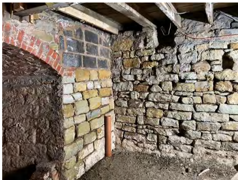
The east wall showing the junction with the north wall and the difference in the masonry between the two walls
