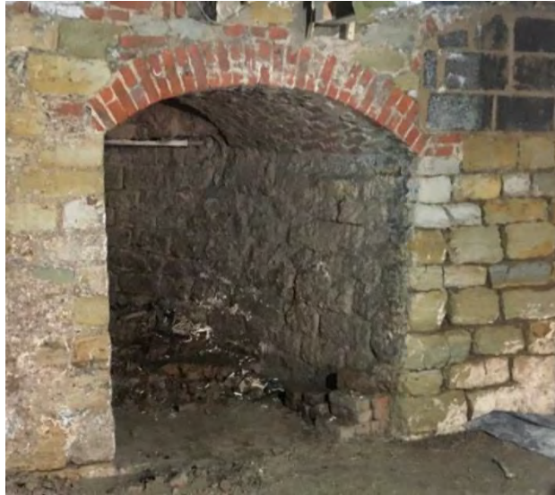
The arched feature at the east end of the north wall. Note the batter on the side walls to the opening more pronounced on the eastern side
