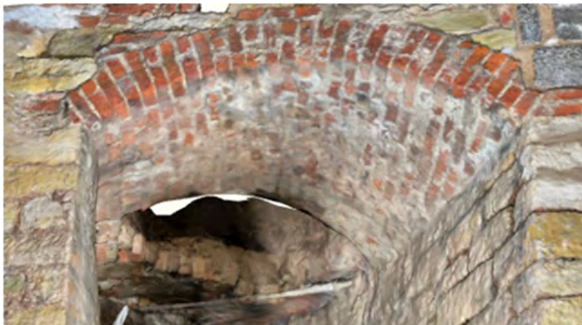
Arch detail showing the skew at the east (right) end
